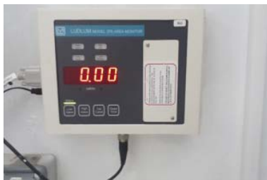
Fig. 12. Radiation monitoring system after the upgrade.
