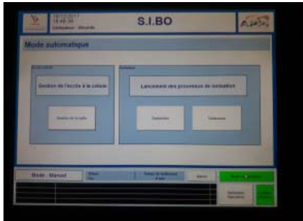
Fig. 11. Operation panel of the control system after the upgrade.
