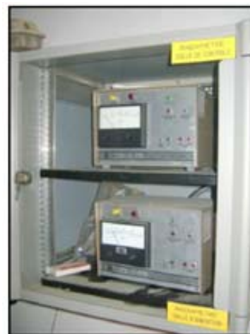
Fig. 2. Initial radiation monitoring system.
